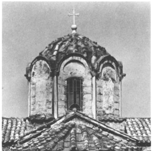
54. The Dome before Restoration. Alternate windows had been blocked up and the arches of the others lowered and flattened.
